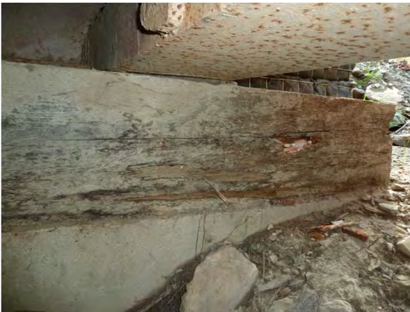
Figure 1-19: Woods end upstream bearing (note sap rot on exposed portion of timber).
