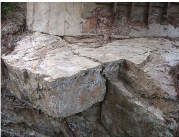
Figure 1-15: Fractured rock below camp end abutment.
