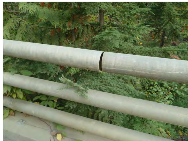
Figure 1-10: Missing railing splice near woods end upstream side.
