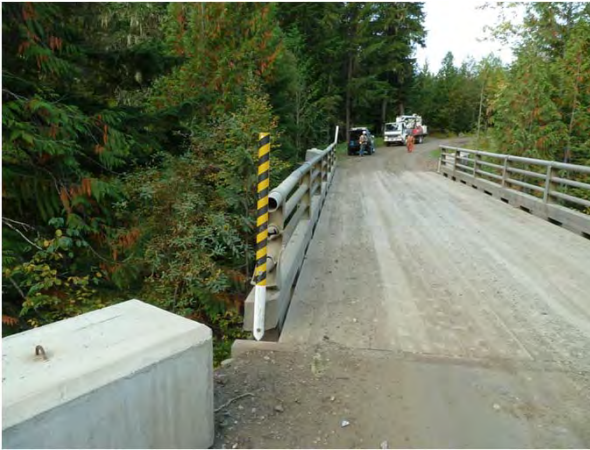
Figure 1-7: Incorrect delineator, woods end downstream corner.
