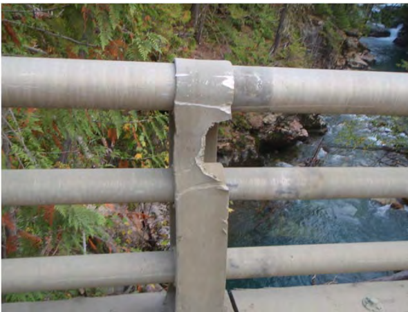
Figure 1-11: Damaged post near camp end upstream corner.
