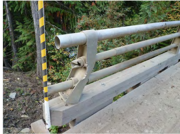
Figure 1-8: Damaged end, post woods end downstream corner.
