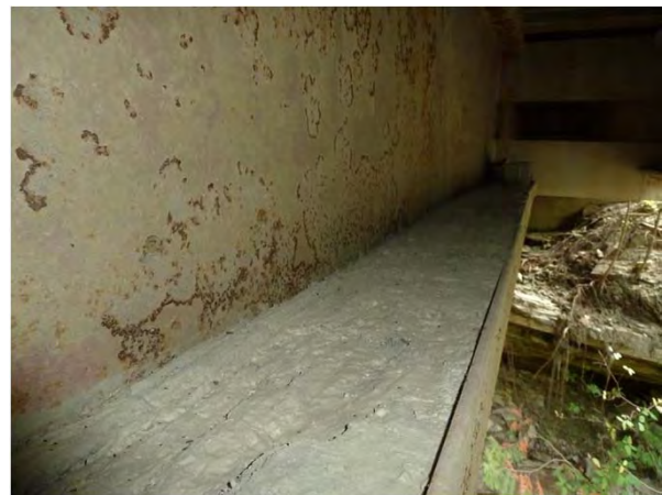
Figure 1-22: Debris accumulation on bottom flange.
