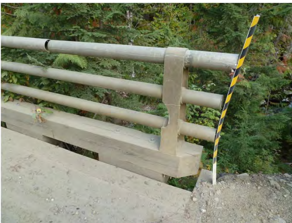
Figure 1-9: Damaged post, woods end upstream corner.
