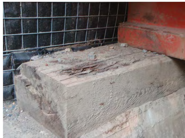
Figure 1-16: Camp end downstream timber sill (note pocket of rot).
